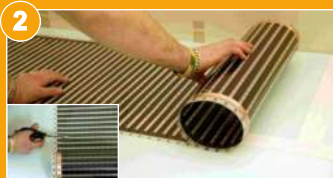
Roll out the ECO FILM SET elements and trim to length along the cutting line as required.
